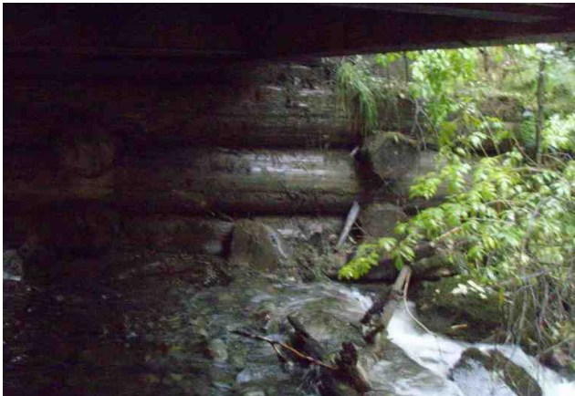
Figure 1-16: Woods end log crib downstream end.
